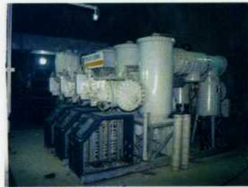
Gas Insulated Switch Gear
