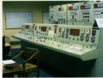
Powerhouse Control Room
