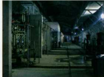
Underground Transformer Hall
