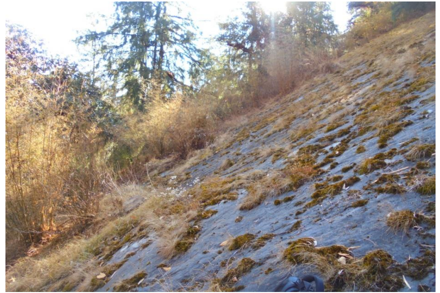
Rock exposure of Quartz rich Biotite muscovite Gneiss at Adit portal 1 at near Nadun Village (Alternative 2(A))
